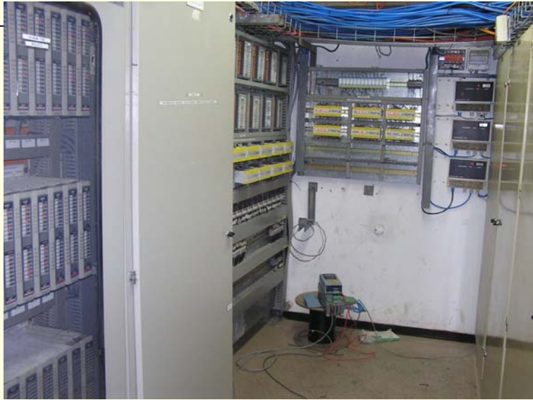
Electrical Room Demux Rack for R-01/2 & S-02 Line Production
